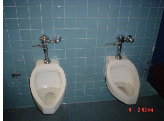
Flush volume on trough-like urinals above can not be reduced to less than 1.5 gpf. Water use can only be lowered to 1.0 gpf or less by replacing the china.
