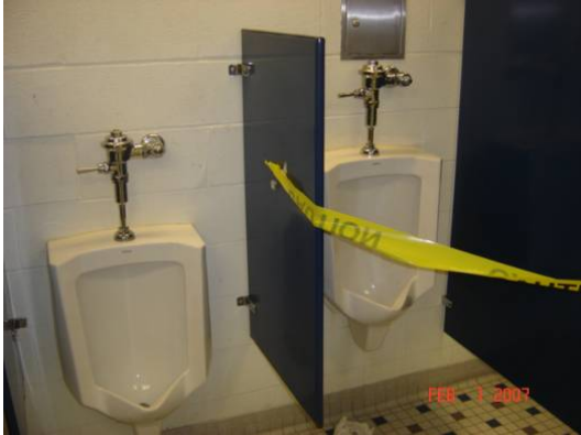
This urinal was closed off because the diaphragm valve continued to run. Valve needs to be replaced.
