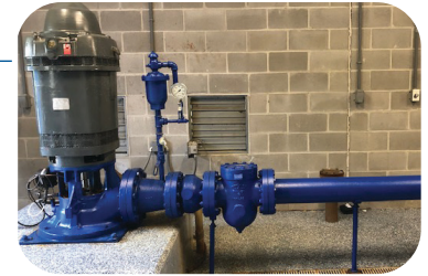
A typical University of Connecticut Well Facility
